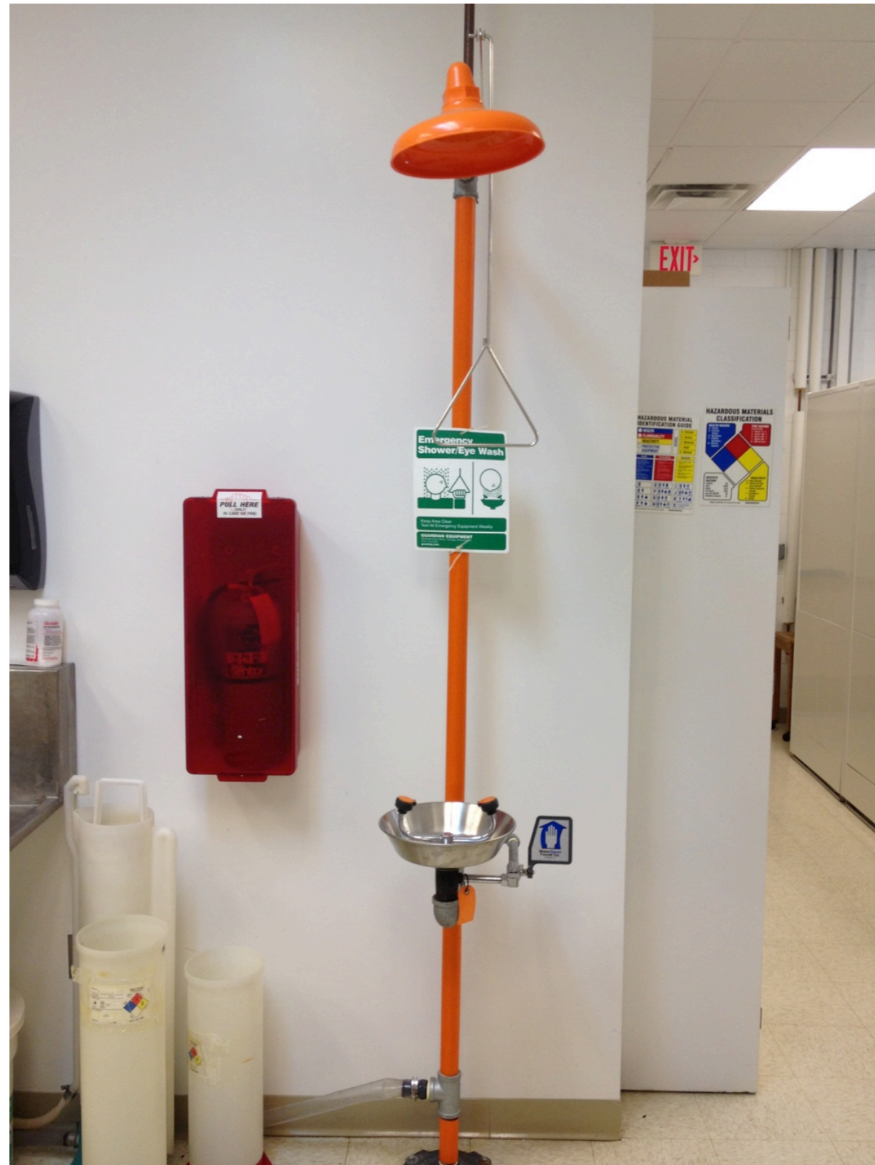
Safety Station with emergency shower/eye washer
