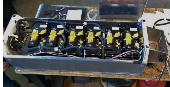
Figure 4: The aluminum battery container houses 6 batteries, and is located on the top of the tunnel.
